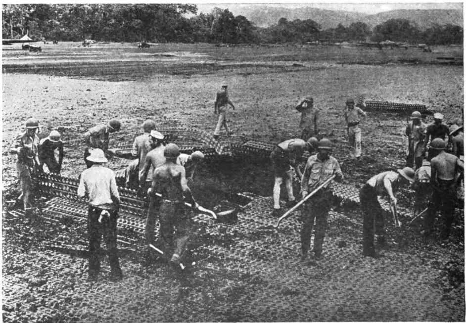
Figure 102. Steel landing mat damaged by bomb hit.
